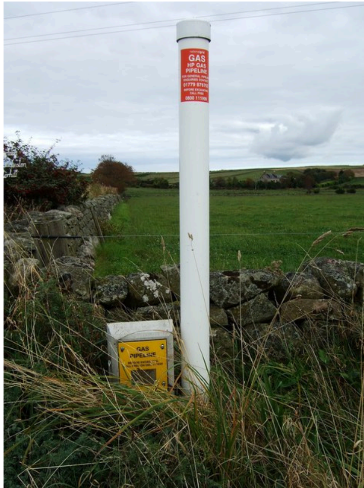
Example gas pipeline marker, Google
