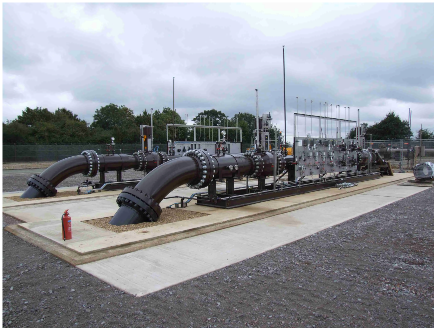
Example of an Above Ground Installation, Google
